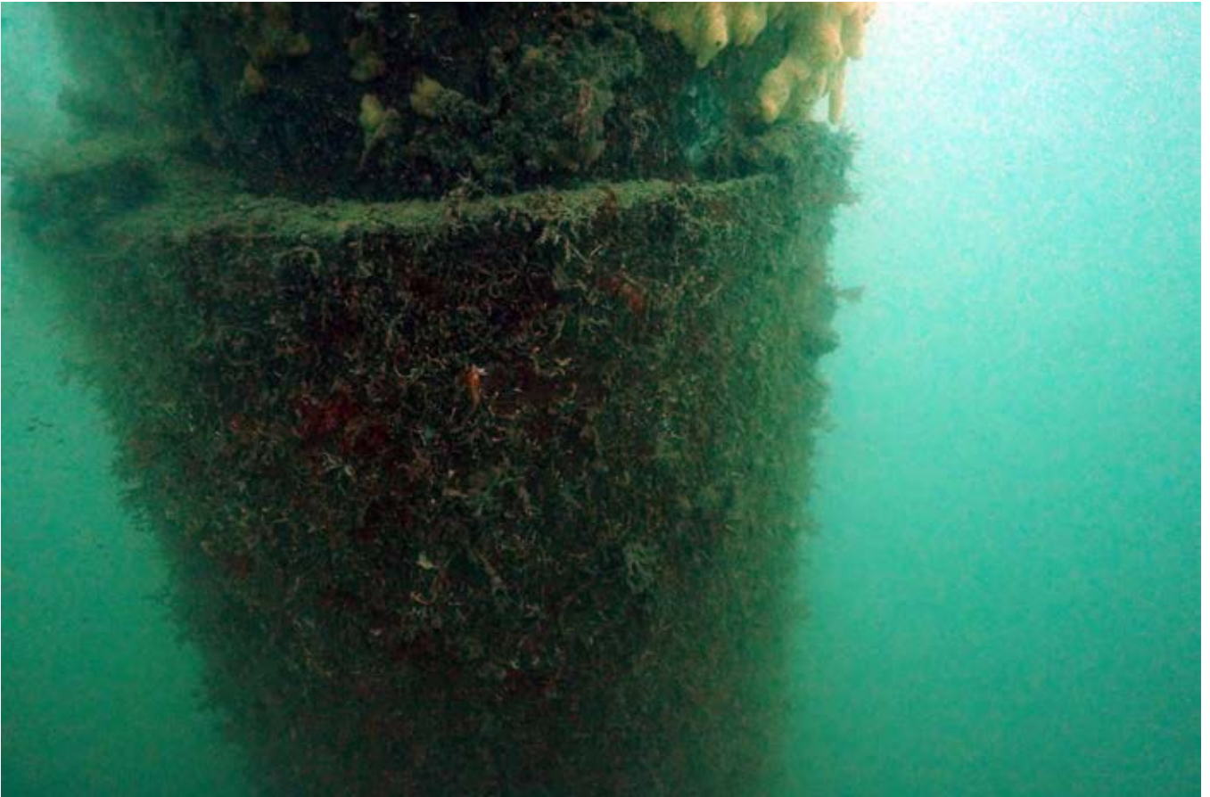
Figure 6: FRP jacketing of deteriorated timber pile – seabed installation – marina general berth position
