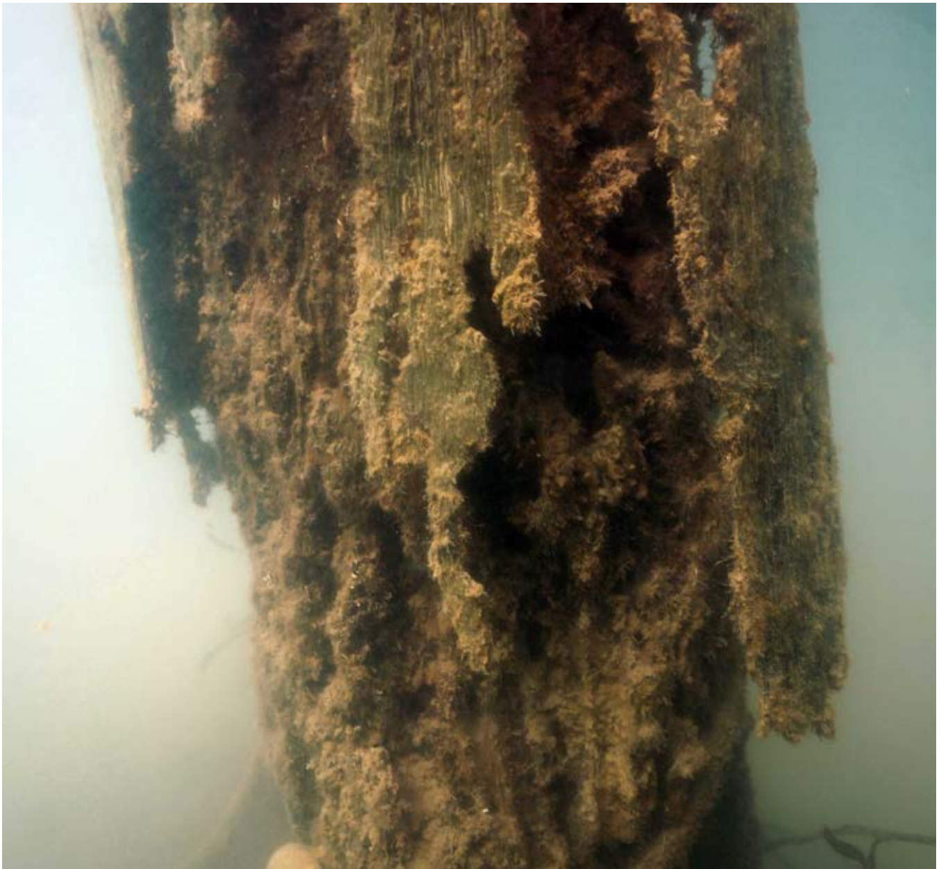
Figure 1: 'Pinus Radiata' timber pile exhibits clear evidence of 'Limnoria' borer damage
