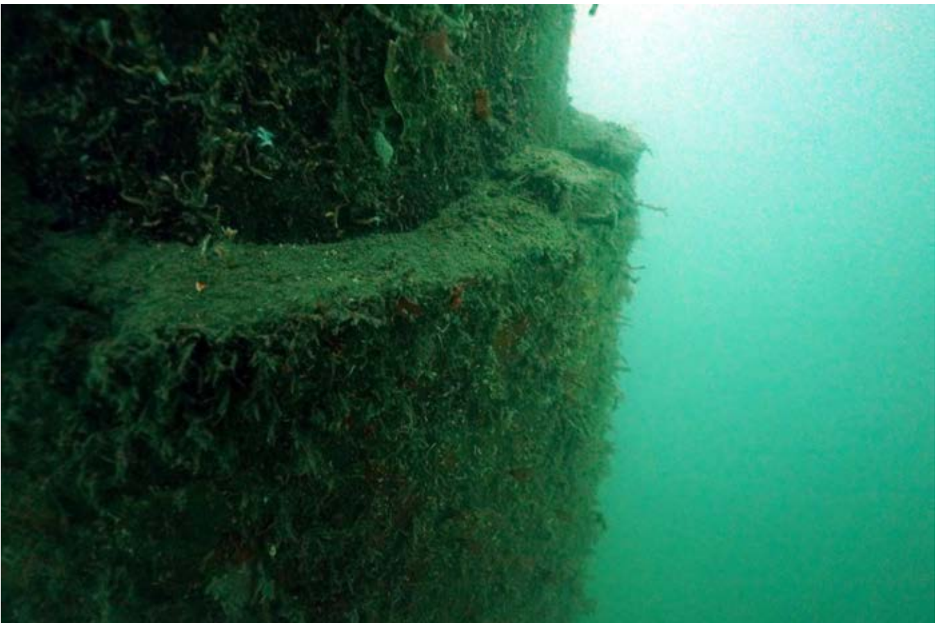
Figure 7: FRP jacketing of deteriorated timber pile – seabed installation – marina general berth position
