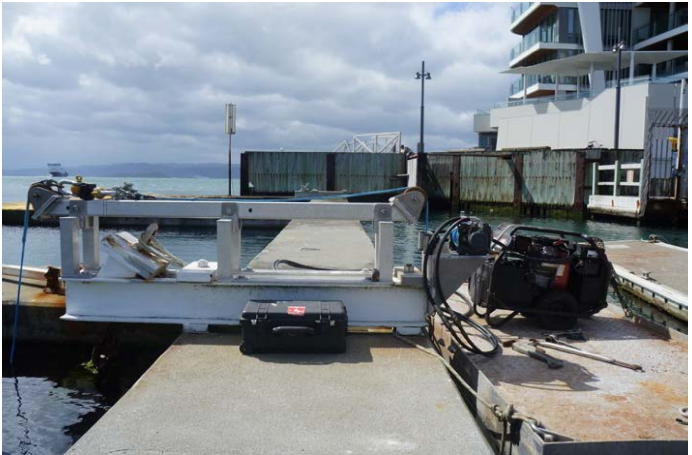
Figure 10: UCL custom built a load testing and pretensioning system for the purpose of checking wear in old chains; installation and setting pretension of new chains
